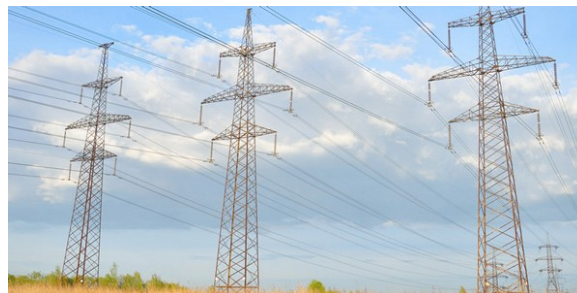
Source: Pacific Gas and Electric
